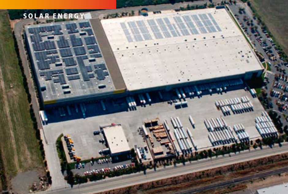
Fig. 5: Distributed solar: Sun-Edison 1 MW PV installation in progress on a Walgreens in Woodland, CA, USA
